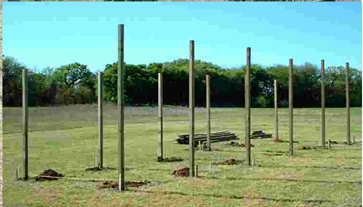
What was accomplished? 1 Mowed Field, 12 set poles, and a pile of free lumber. Great work STRCC! Let's keep it going! I want to fly soon!
