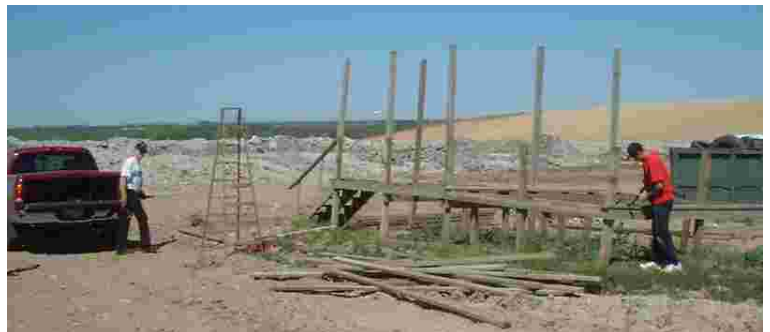
Mario and Joe are doing some demolition. This wood will be used on the new shade awnings
