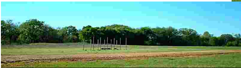
C and D added some more dirt to the runway and packed it down. All we need to do is to smooth it out and put on the petramat! I think STRCC owes C and D a Barbeque!
