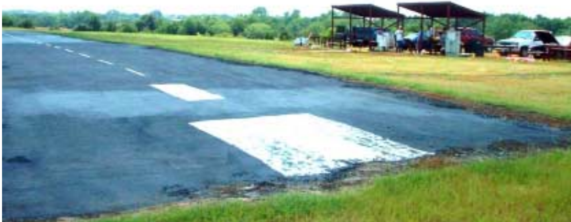
The runway resurfacing project is officially complete. Stripes have been added and it looks great! I would like to thank all of those who helped out!
