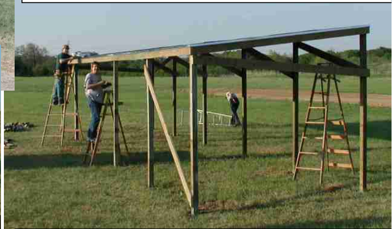
All is in place for the shade – A retreat from the heat!
