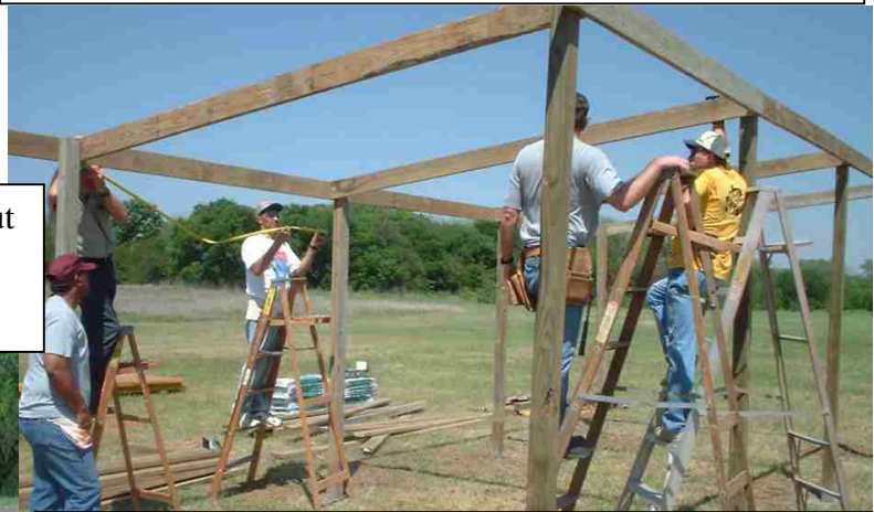
A few more timbers are in place before the roof goes on.
